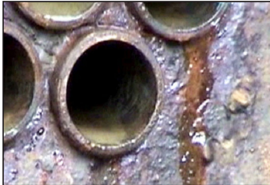
Original condition of the tube sheet
